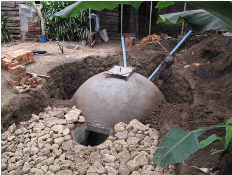
A dome-type biogas digester under construction in Arusha, Tanzania. Image: Laramie & Davis (2013)
